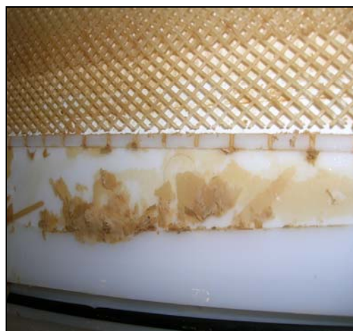
Figure 5. Scale formation blocking the distribution channels
